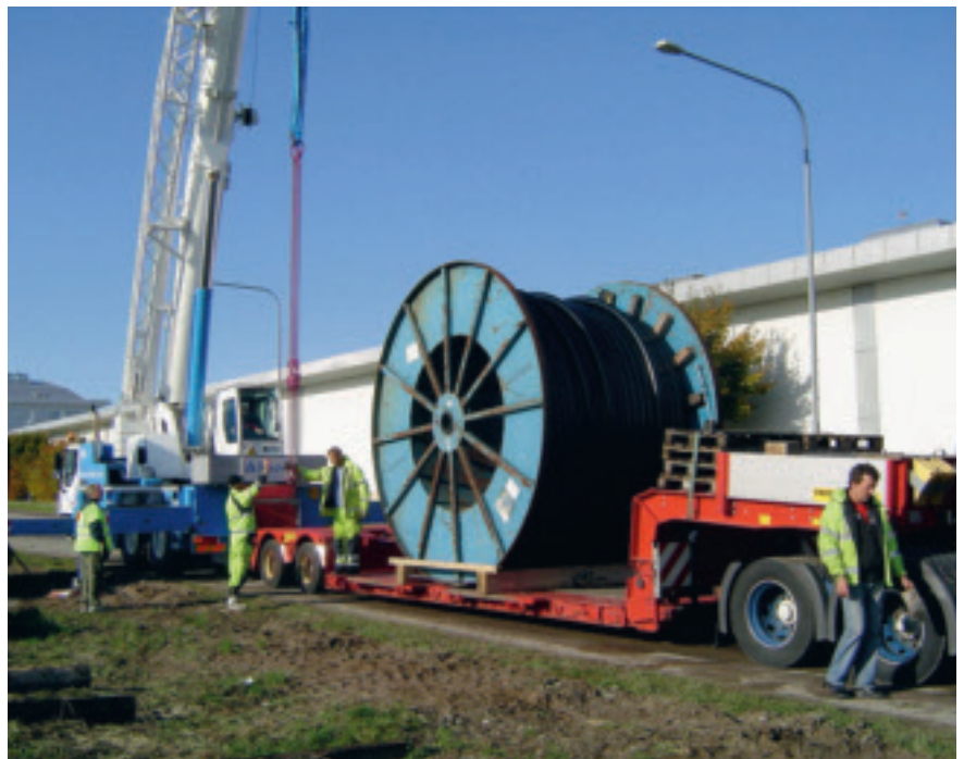
The 220 kV cables that will provide a new feed for Uppsala were delivered in November 2008, thereby strengthening the supply to the city.
