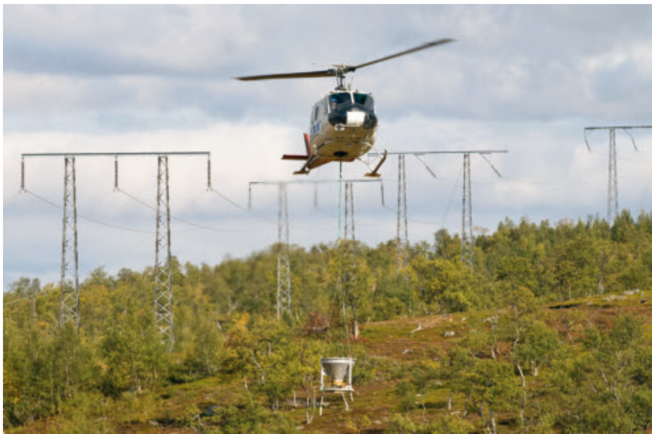
The work of building the Swedish part of the new 400 kV powerline between Järpströmmen and Nea started during the latter part of 2008. A large proportion of the material was flown in by helicopter.
