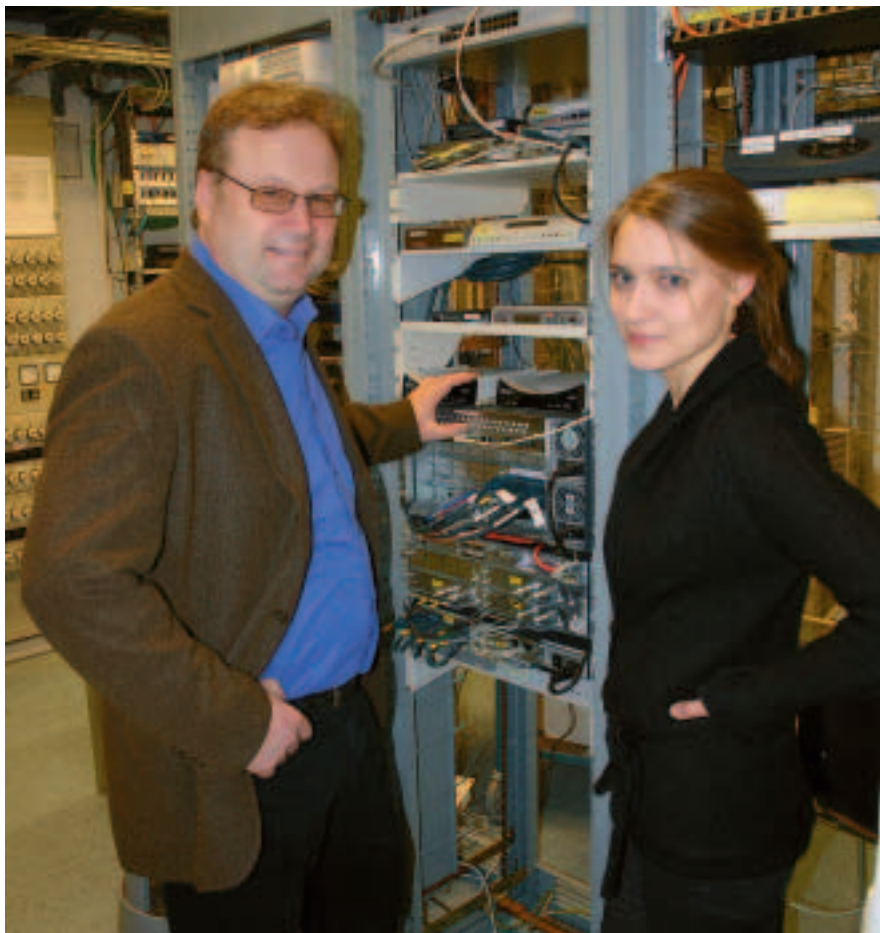
Svenska Kraftnät collaborates with Vattenfall Eldistribution, among others, with regard to issues that involve telecommunications.
