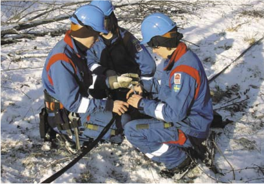
Hurricane Gudrun disrupted the electricity network in the south of Sweden, but the 400 kV and 220 kV national grid power lines remained intact. Svenska Kraftnät helped the electricity companies to restore electricity supplies, among other ways by lending out equipment and contacting people who had previously been trained as linemen at our training centre in Åsbro.
