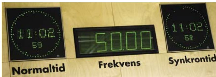
Svenska Kraftnät makes sure that the frequency in the power network remains at 50 hertz.
