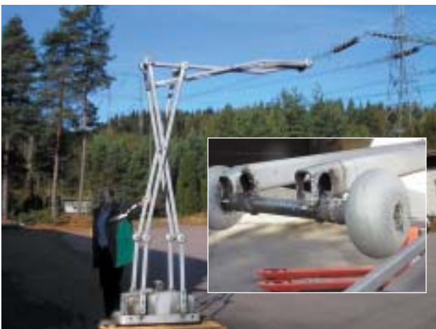
When the isolator at the Horred station failed, an arc arose which short-circuited parts of the switchyard. The damage to the isolator can be seen in the inset picture.
