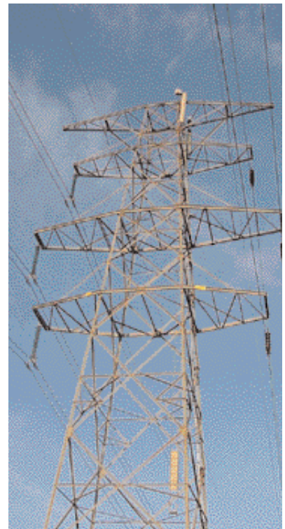
A GPS antenna has been fitted to one of Svenska Kraftnät's pylons at Viksjo outside Stockholm.
