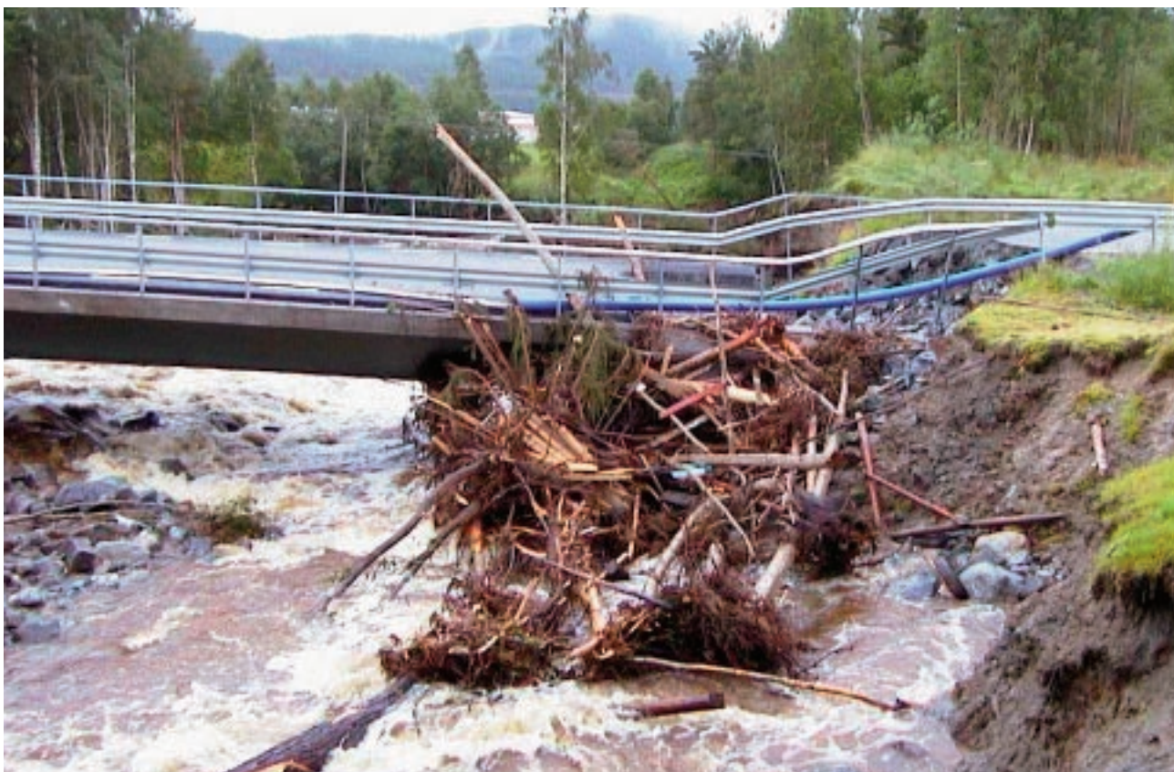
Damaged bridge over an unregulated river in northern Sweden.
