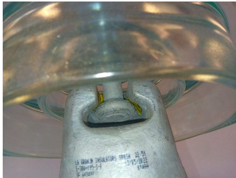
Figure 10: Yellow and green insulator tape separating the top bell from the bottom bell
